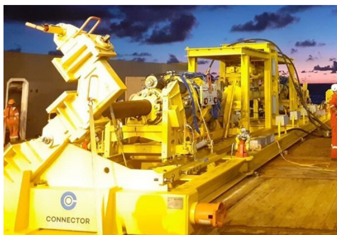
SSIV Skid mounted with diverless connectors, awaiting installation
